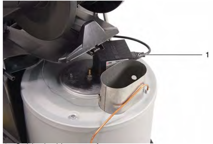
1 Cable, ignition transformer
